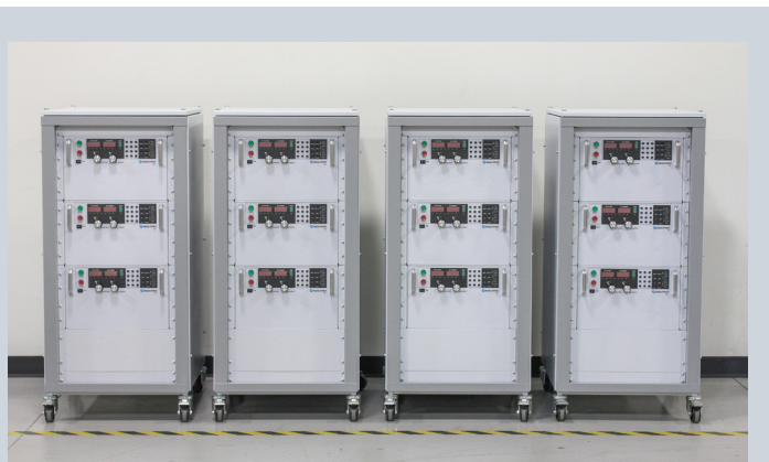
Qty (12) 30 kW TS Series with water cooling (+WC) packaged in Qty (4) CAB2
